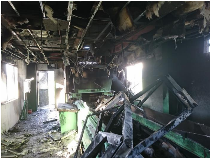
Fire caused by LiB crushing at recycling facility
